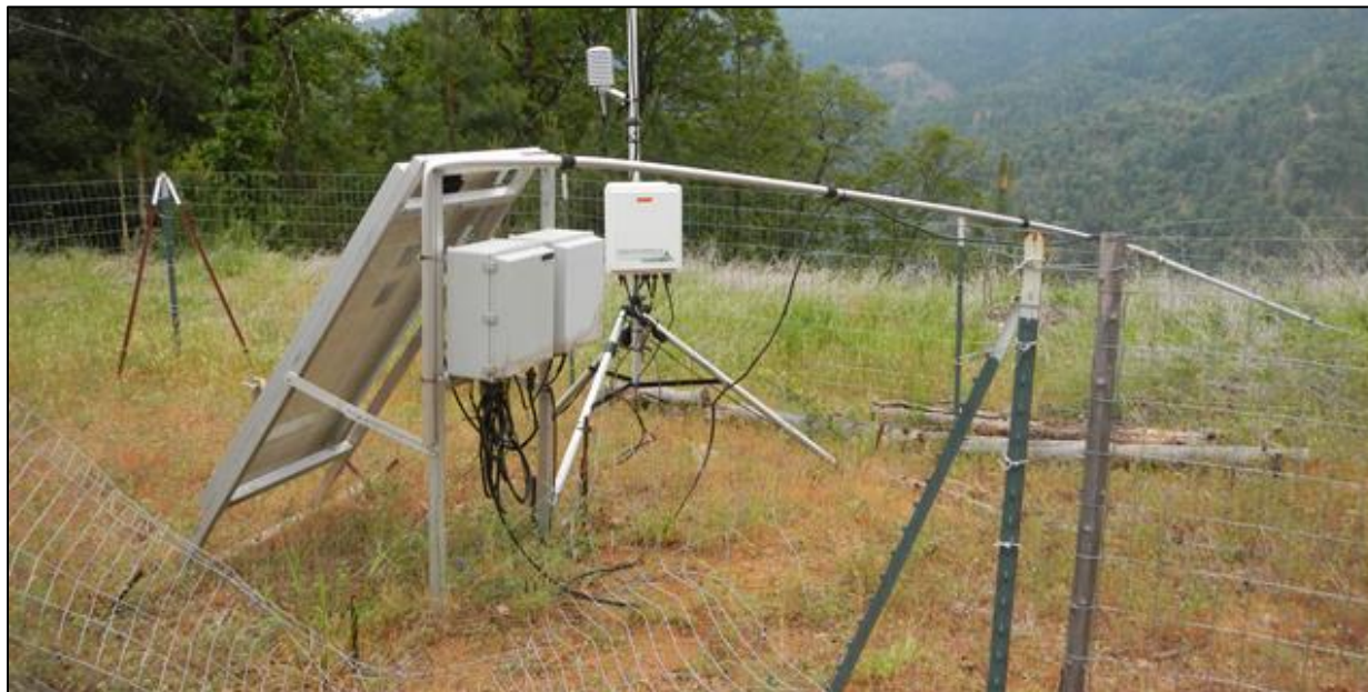
Figure 13: Weather Station with Bear Damage
